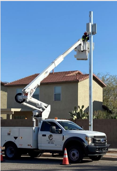
Verizon small-cell pole
