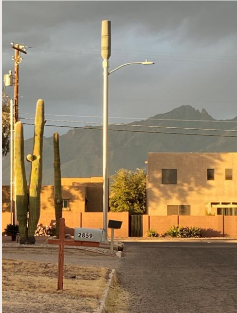
AT&T small-cell pole
